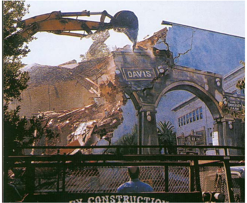
The demolition of the Terminal Hotel Building and the Arch Mural on the North wall. This picture taken from the cover of John Lofland's book, "Demolishing a Historic Hotel. A Sociology of Preservation Failures in Davis, California." It is rather graphic by itself.
